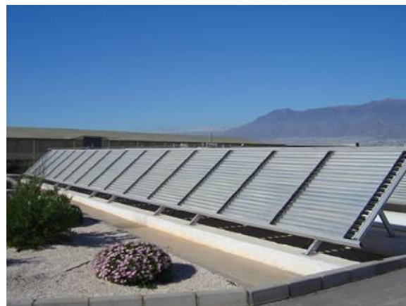
Fig. 1. View of one of the rows of the solar collector field.
